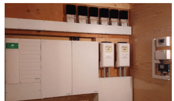
Viridian's micro-hydro load diversion or "dump load" arrangement, using six Morningstar TS-60A controllers
