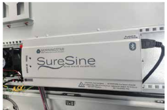
Morningstar’s SureSine inverter and charge controller efficiently and reliably produce the AC electricity needed to keep the communications tower operating
